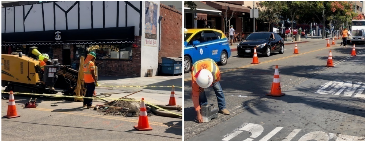
Figure 2. Horizontal Directional Drilling. The tech at right is tracking the drill head and looking for underground utilities. (source: FOA)
