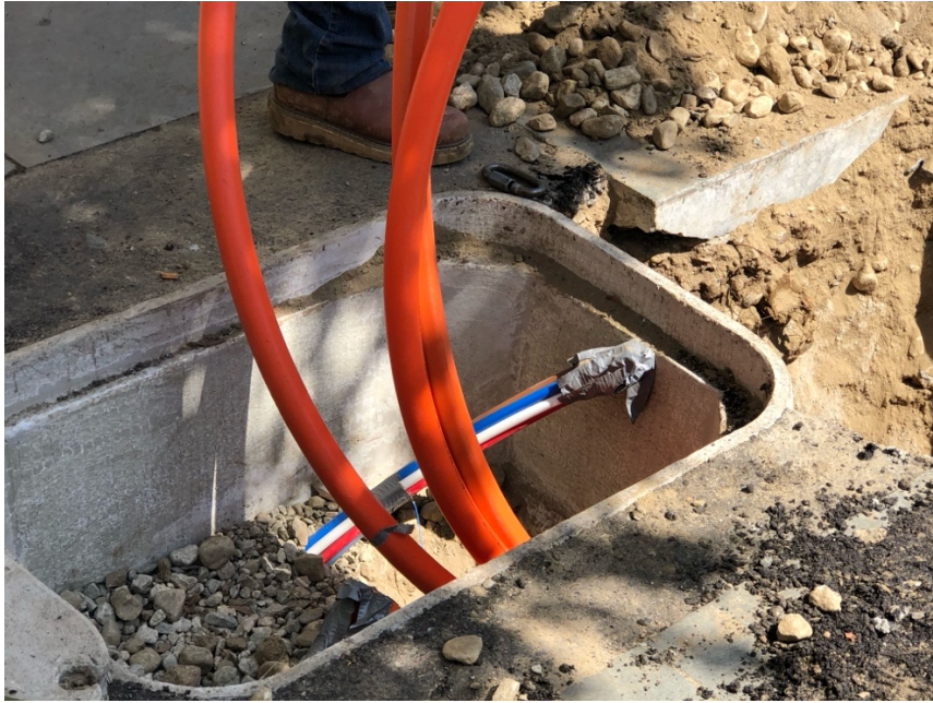
Ducts and microducts in the same handhole
