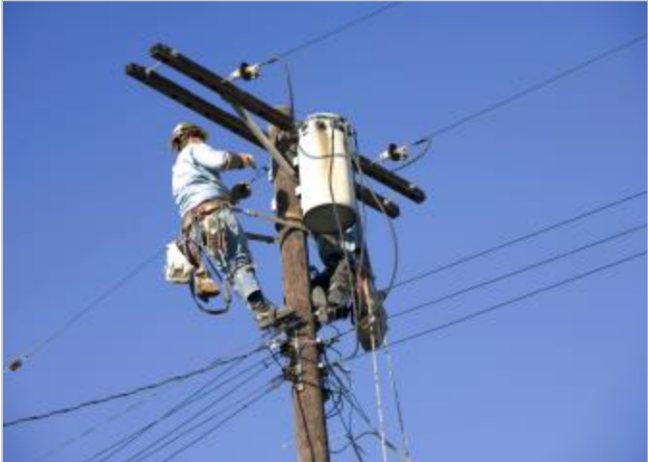
Line installers and repairers often work in teams to install and fix cables and wires.
