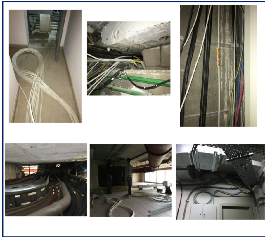
Riser Cable Laying From the roof top to the shared Telecom room and step transitions
