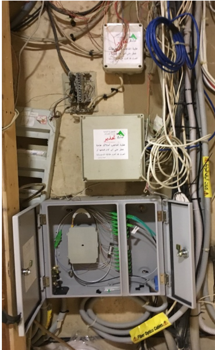
Photo (Left) shows FTTH BDB adjacent to legacy PSTN infrastructure. Clear identification of FTTH wiring essential.
